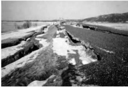
Fig. 1. A failed embankment in the 1993 Kushiro-oki Earthquake (Fudo 1994)
